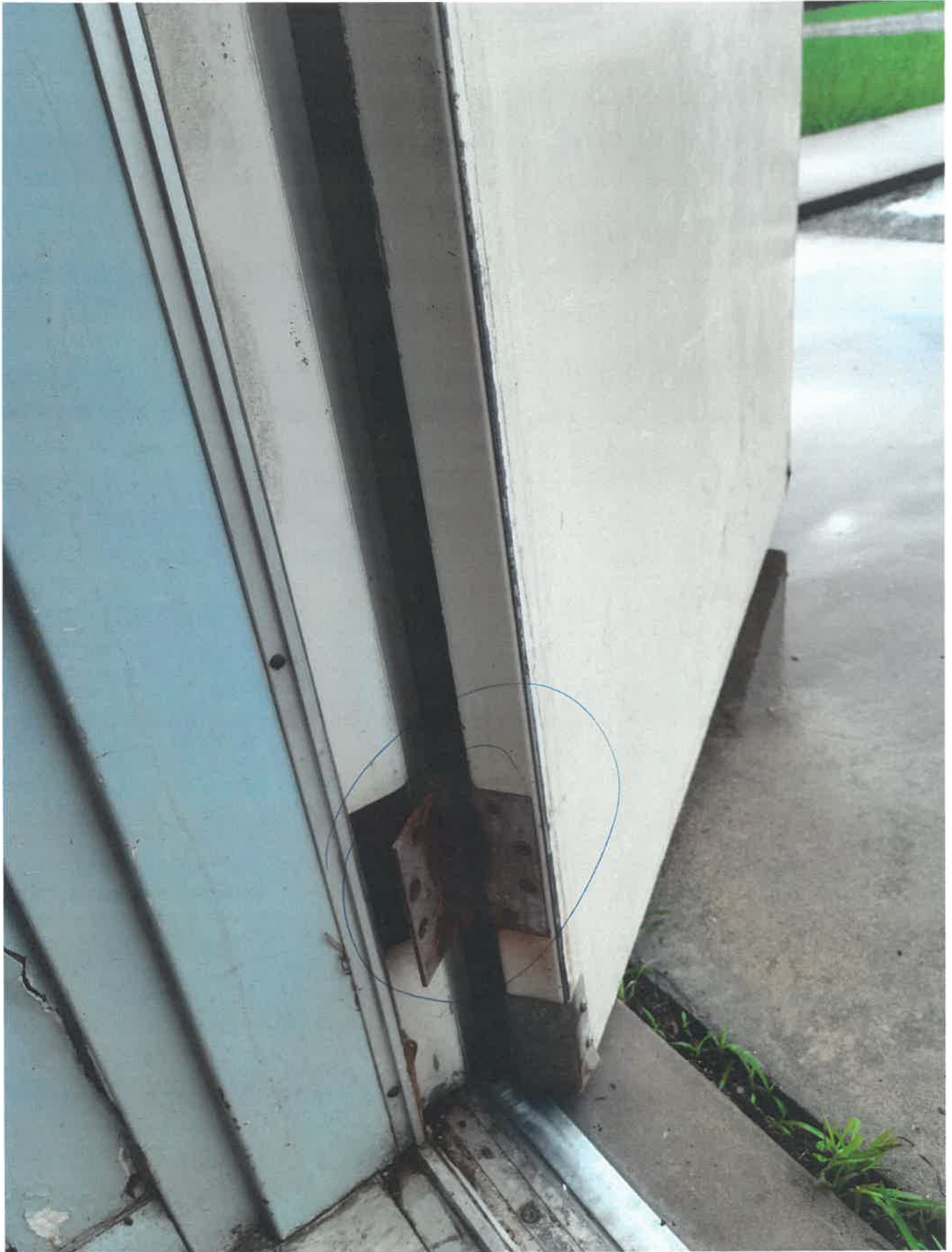
Rusted Hinge on Kitchen Entrance (All Hinges on exterior are rusted out)
